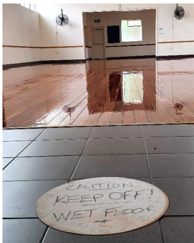
Coles Hall renovation: The newly-sanded floor after the second coat of sealant.
